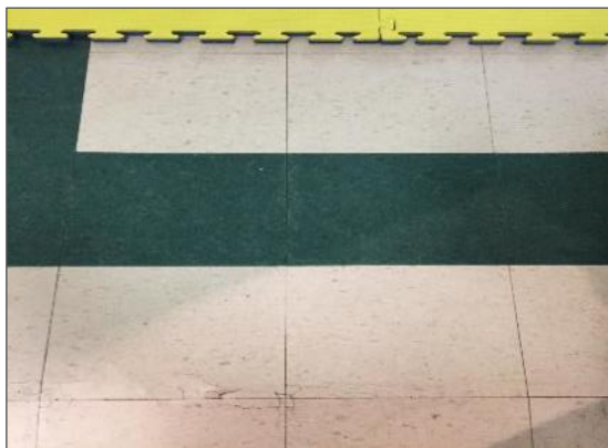
Photograph No.10: Non-asbestos vinyl floor tiles in the basement yoga room Loc. 9 (Samples 0012A-C).
