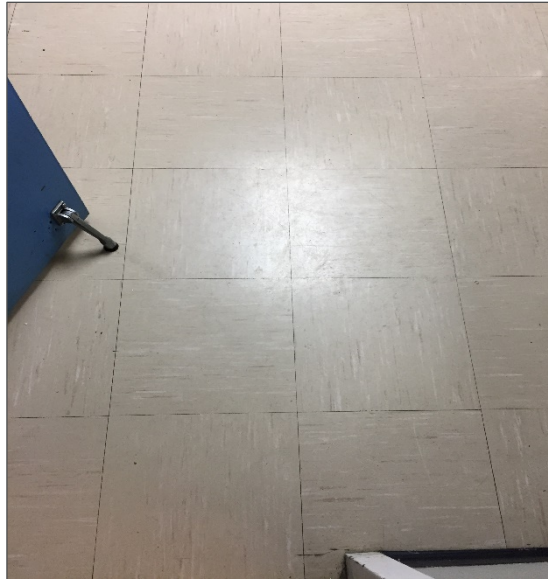
Photograph No. 18: Asbestos-containing vinyl floor tiles within the staff room Loc.59 (Samples 0046A-C).
