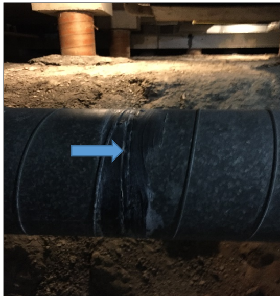
Photograph No. 23: Non-asbestos black/grey mastic present on uninsulated ducting within the south crawlspace and basement (Samples 0005A-C).
