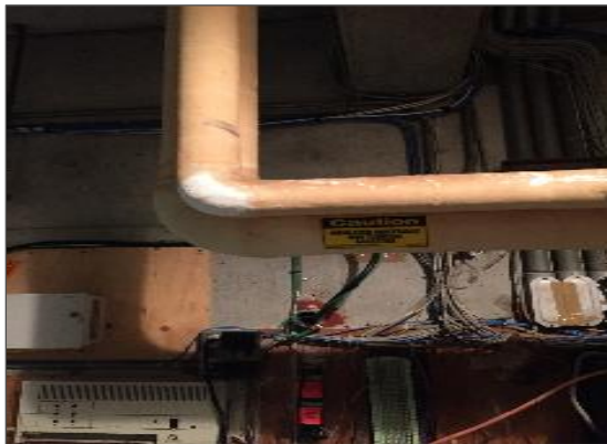
Photograph No. 1: Asbestos-containing parging cement present on fittings, elbows, valves and tee's of the Domestic, hot water, steam system.
