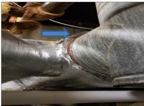
Photograph No. 21: Non-asbestos red/brown mastic on uninsulated ducting within the basement (Samples 0003A-C).
