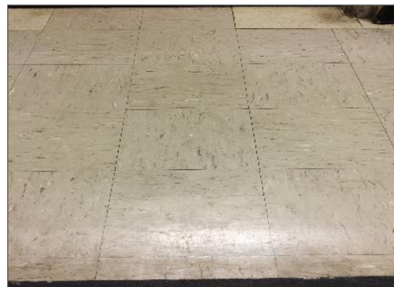
Photograph No.11: Asbestos-containing vinyl floor tiles Various Locations (Samples 0015A-C).
