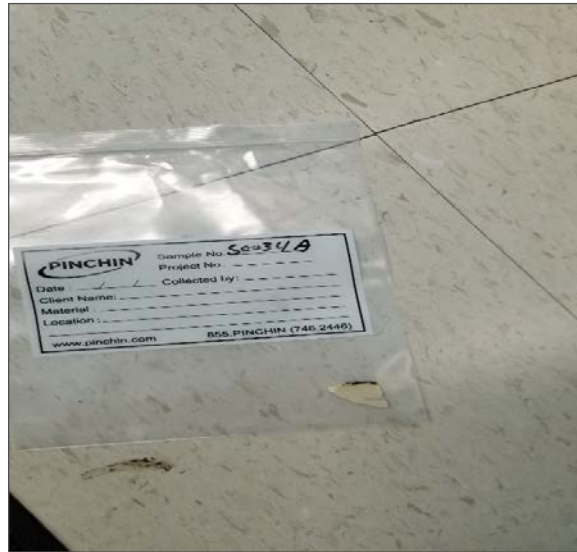
Photograph No. 14: Non-asbestos vinyl floor tiles within the pool corridor Loc.38 (Samples 0034A-C).
